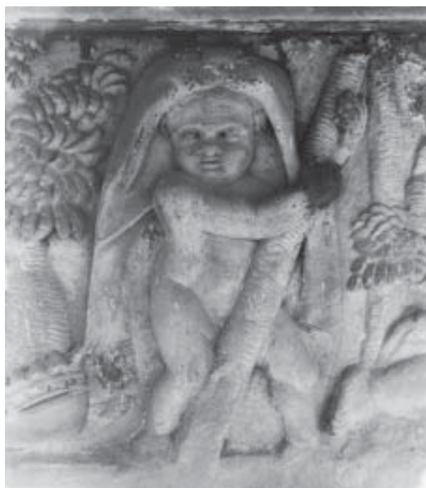
3. Anton Povolný: County House in Levoča, 1807 – 1826, detail of the sculptural decoration, relief with putti. Repr: Documetation to the restoration , 1997.
